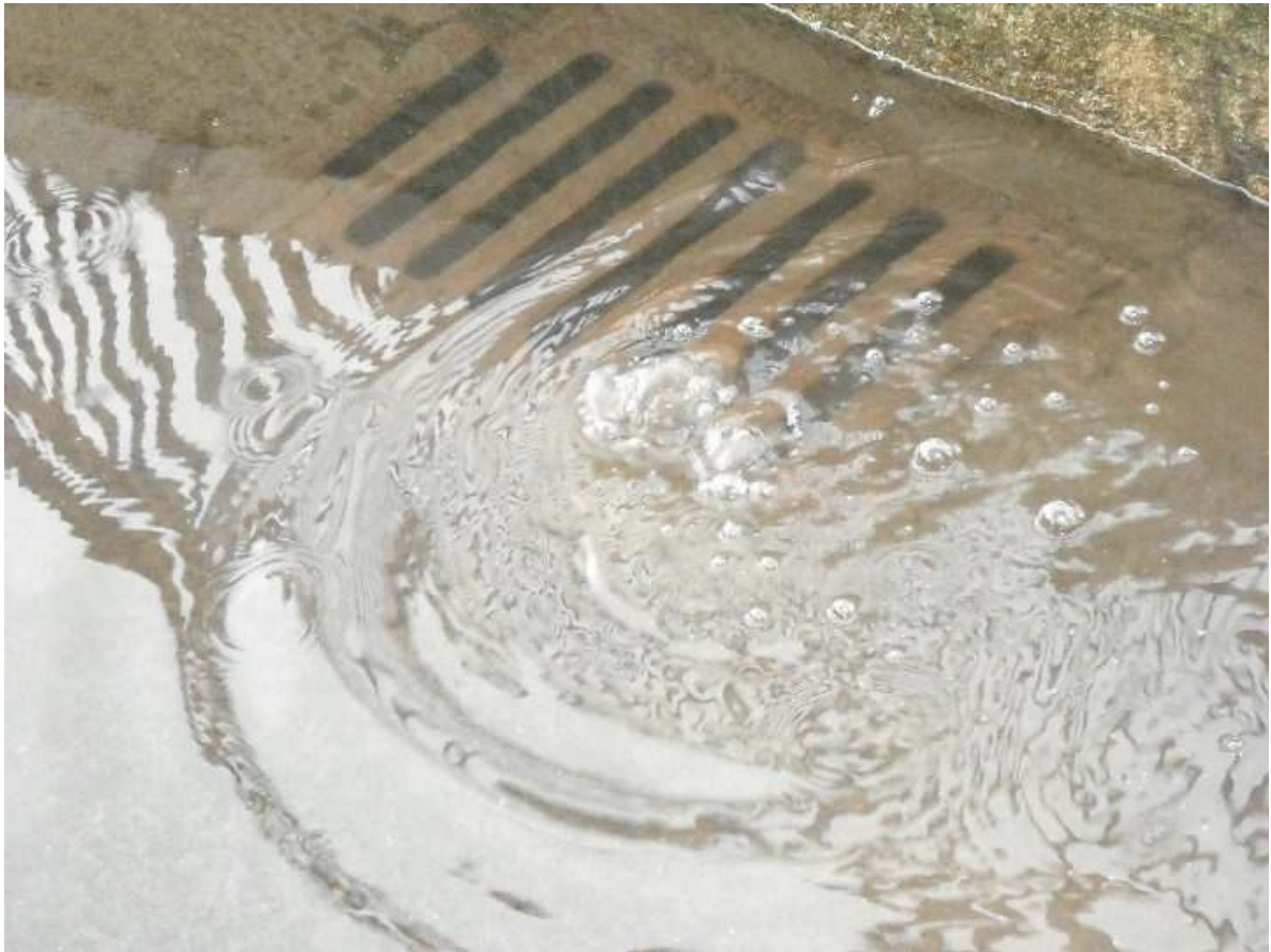
Bennetts Walk 7 th July 2009 The gully is clean but the drains cannot carry the water away
