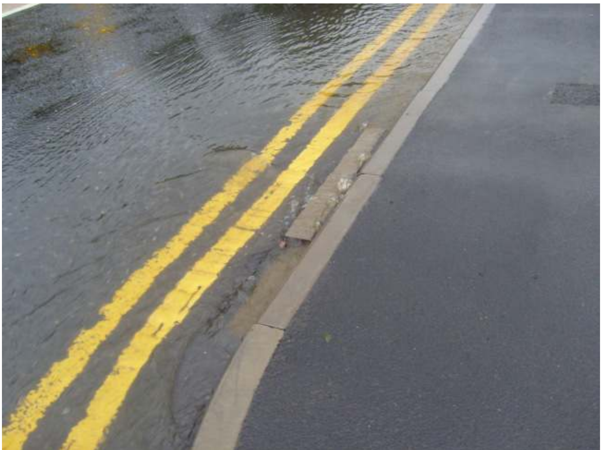
The kerb and road surface have been forced upwards by the groundwater The red speck is a trapped frog formerly living beneath the road surface.
