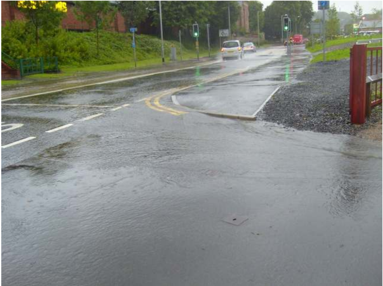
A stream flows from the gulleys and beneath the road surface towards the electricity substation 17 th July 2009
